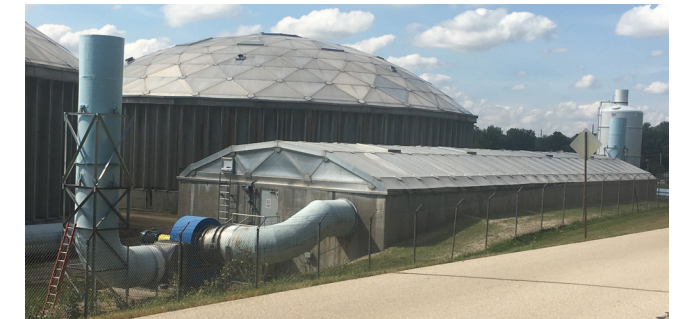
Cedar Rapids Biofilter System
