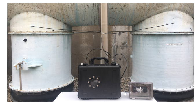
Field Sample Collection from the Two Biofilter Inlet Ducts
